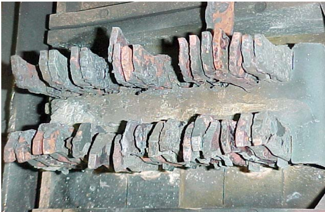
Fig.2. Finger Cluster after failure in July 2000
