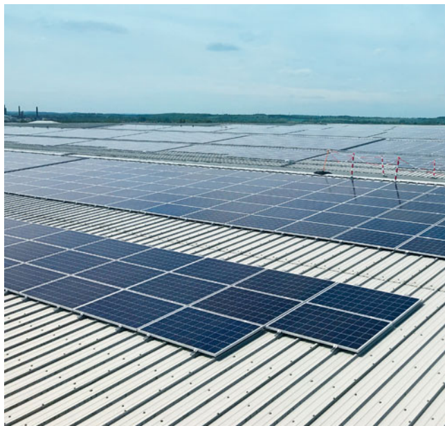
1,000 kW solar PV installation at our distribution centre in Newark let to Dixons Carphone.
