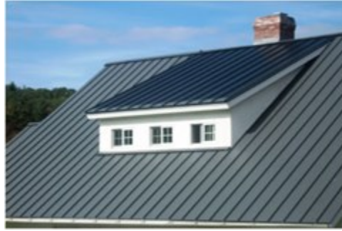
Figure 95-11: Building-Integrated Solar Energy System
